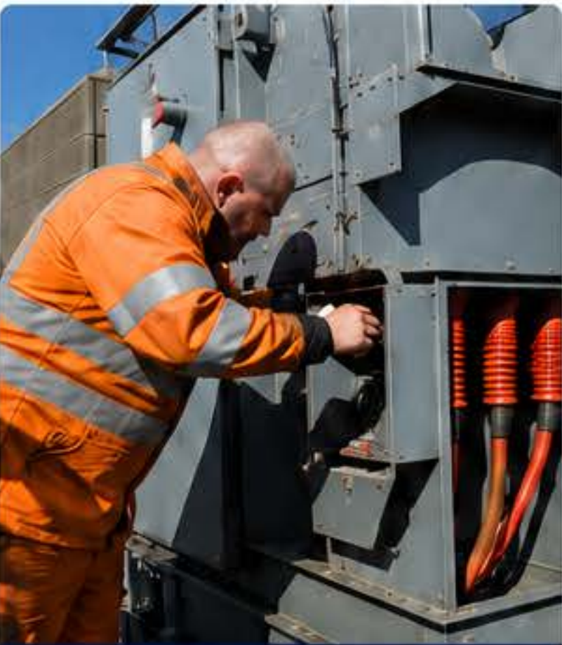
HV EQUIPMENT INSPECTION & MAINTENANCE
