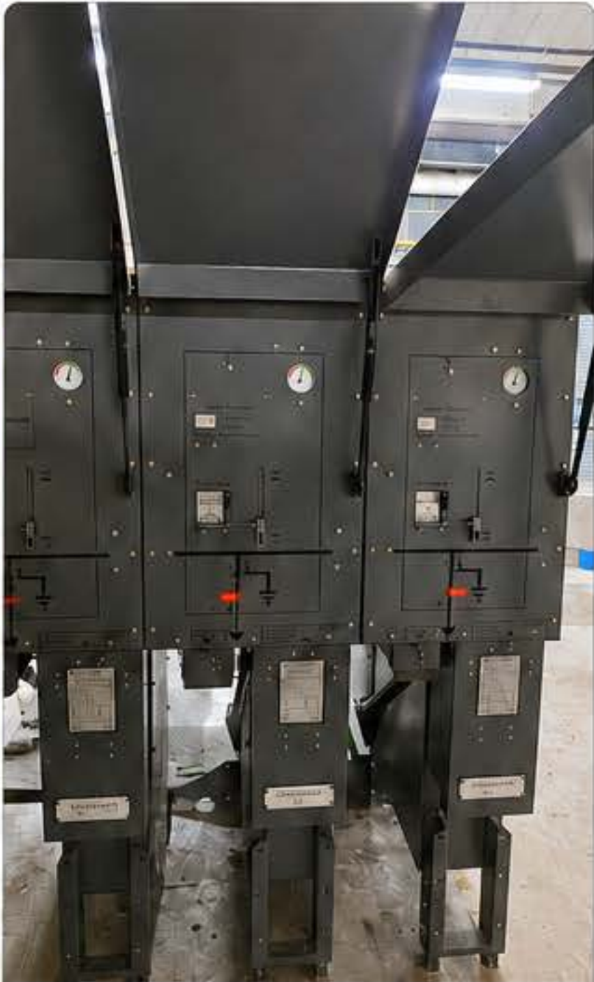
HV CIRCUIT BREAKERS – MAINTENANCE & INSPECTION
